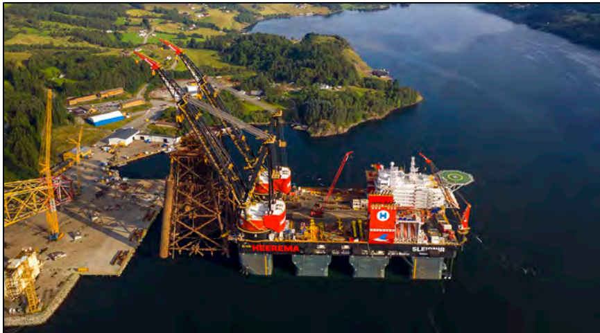
Figure 20. Sleipnir loading Brent Alpha’s upper jacket onto the wharf at AFOD Facility in Norway (Heerema Marine Contractors)
