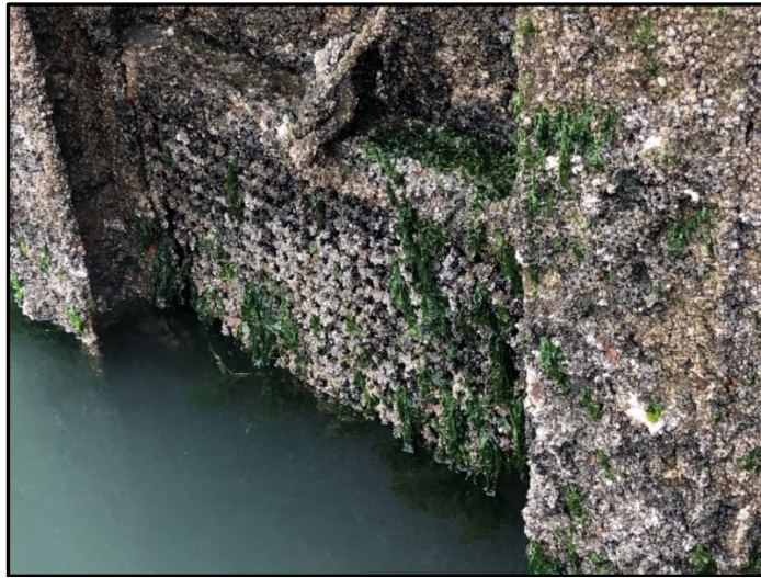
Image 4: Existing water intake screen at the Redwood Marine Terminal II Dock. This screen will be replaced.
