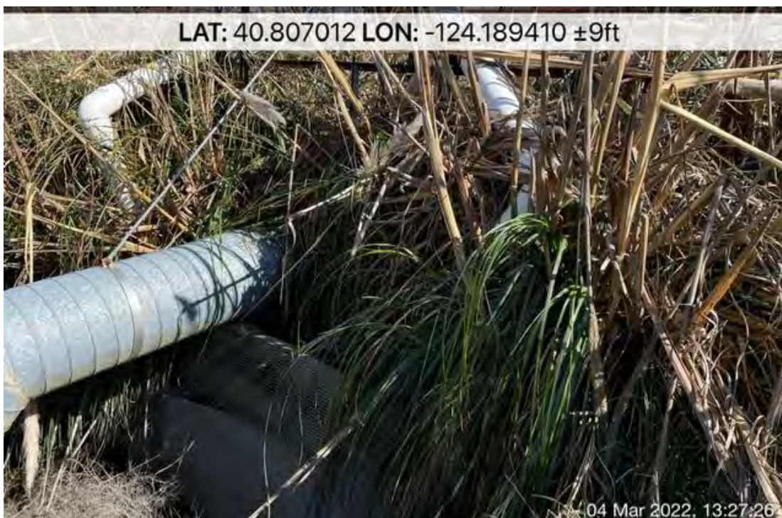
Photo 8: Closeup at existing stormwater detention infrastructure. Note weirs, screening, and overflow pipes. Photo taken March 4, 2022.
