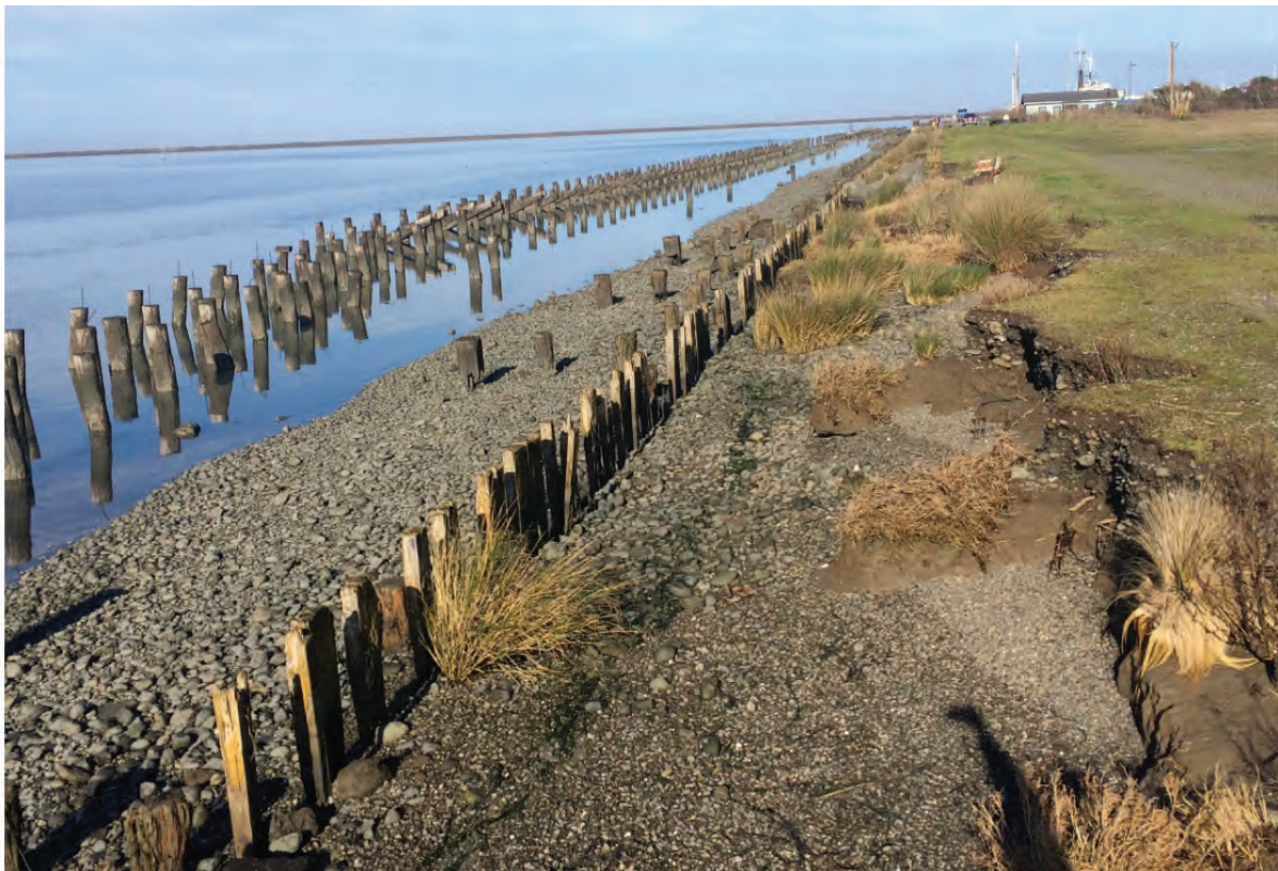
Figure 2. Photo of representative shoreline erosion at project site. Photo source: Stillwater Sciences, 2016
