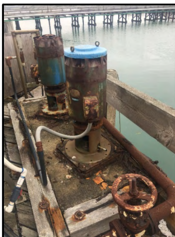
Image 2: Existing water intake pumps at the Redwood Marine Terminal II Dock.
