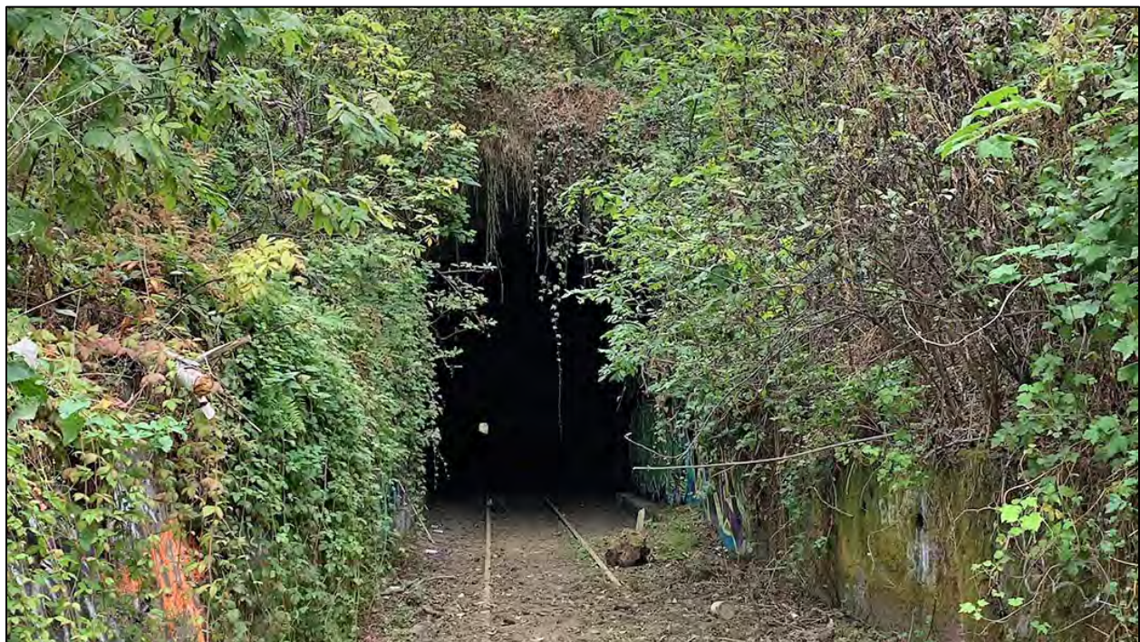
Figure 20. Deferred Maintenance of Tunnel in NCRA Corridor
