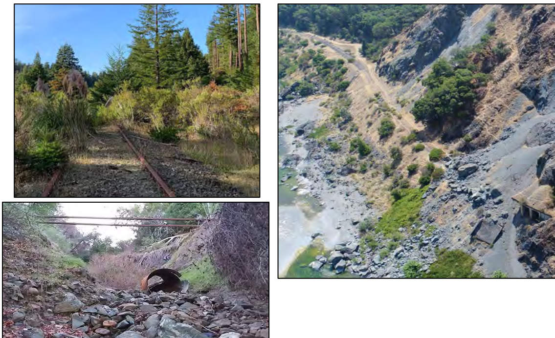
Figure 11. Deferred Maintenance in NCRA Corridor
