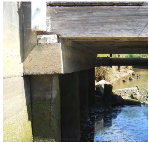
Figure 1: Vertical Cracking on Piles
