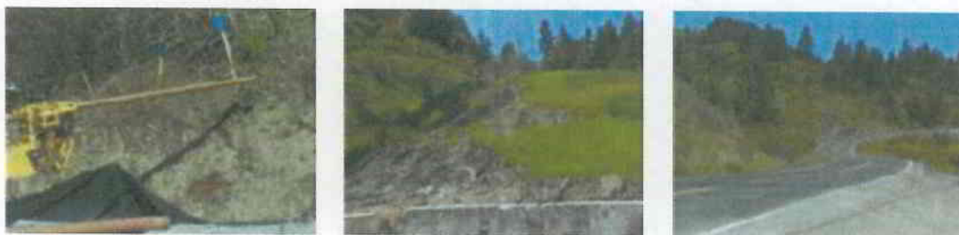
Figure 5 – Photos of Active Landslides Near Proposed Rail Routes
